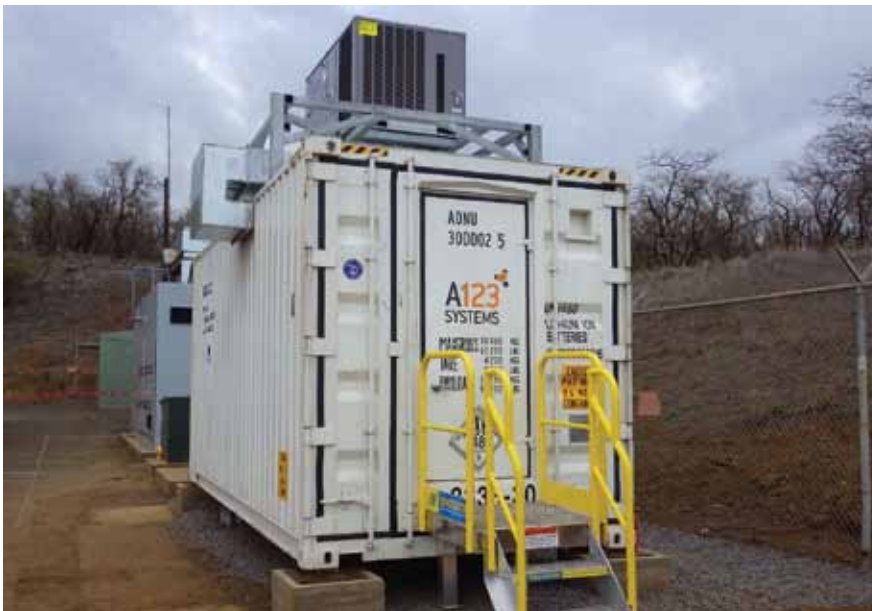
This 1 MW/1 MWh A123 lithium ion battery system at the Maui Electric Wailea Substation, Hawaii, began operating in May 2013. AES Westover and AES Laurel Mountain also use A123 systems. (Photo courtesy of A123 Energy Solutions)
