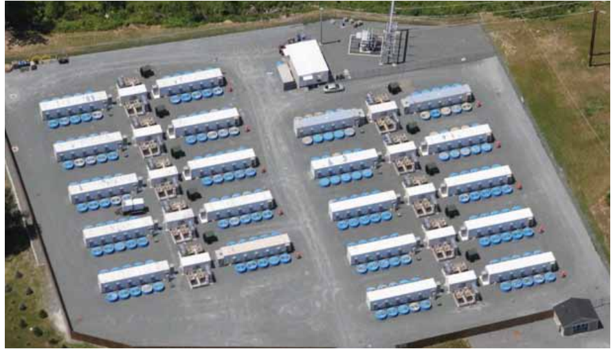
Beacon Power's 20 MW Stephentown Advanced Energy Storage plant. (Photo courtesy of Beacon Power, LLC)
